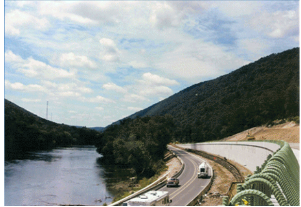
The Lewistown Narrows is impacted by its role as a major transportation corridor, as illustrated here by the widening of SR 322/22.
